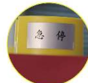
急停开关 Emergency stop switch
