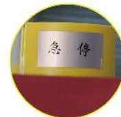
急停开关 Emergency stop switch
