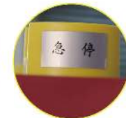
急停开关 Emergency stop switch
